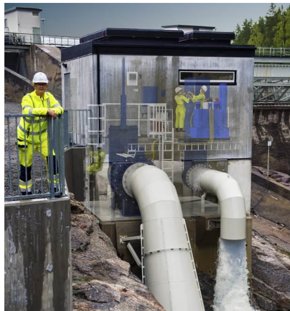
Fig. 1: Gåseflå eco-flow hydropower plant
